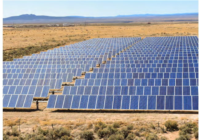
Kit Carson Electric Cooperative solar array.
