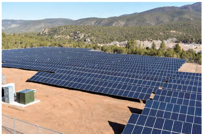
Kit Carson Electric Cooperative’s solar array in Amalia.
